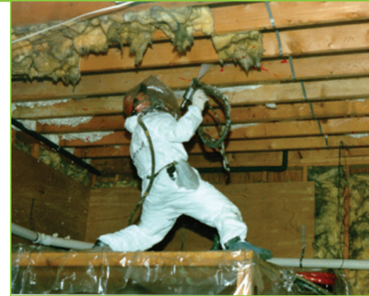
Weatherization staff sprays foam insulation into the home of a low-income client.
