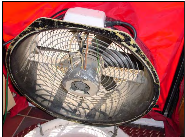
Don't do this! Four small holes in the fan flow sensor ring must be unobstructed and regularly cleared of dust accumulation
